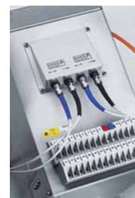
Fig. 5/148 Communication interfaces in a sloped case in a surface-mounting housing
