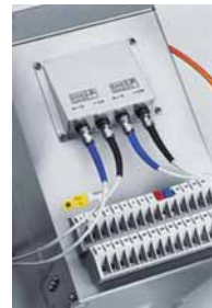
Fig. 10/6 Communication interfaces in a sloped case in a surface- mounting housing
