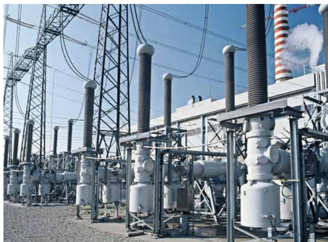
Fig. 2/10 Application in the high-voltage system
