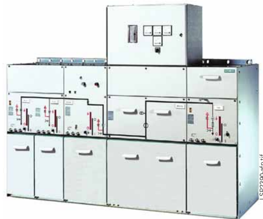
Fig. 5/13 Application in distribution switchgear
