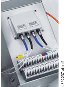
Fig. 6/7 Communication interfaces in a sloped case in a surface-mounting housing
