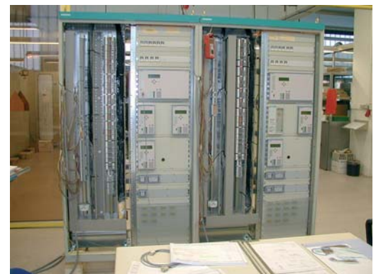
Fig. 8 Testing the generator protection cubicles
