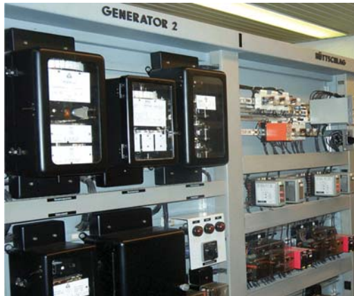
Fig. 2 Existing switchgear panels with protection relays
